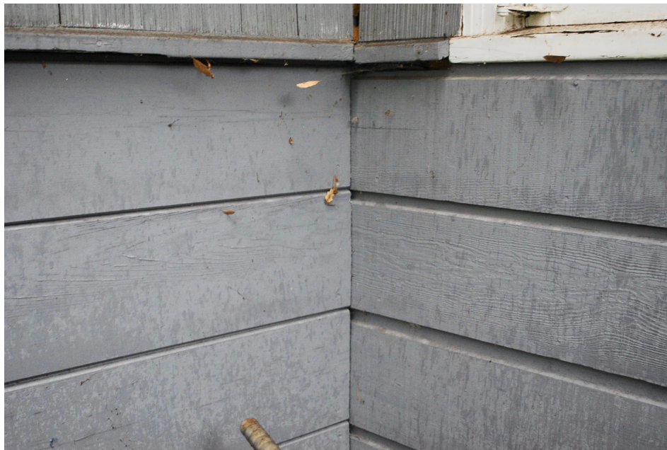
V-groove siding in the base of the south addition (at left) and rustic siding in the base of the main body of the house.
