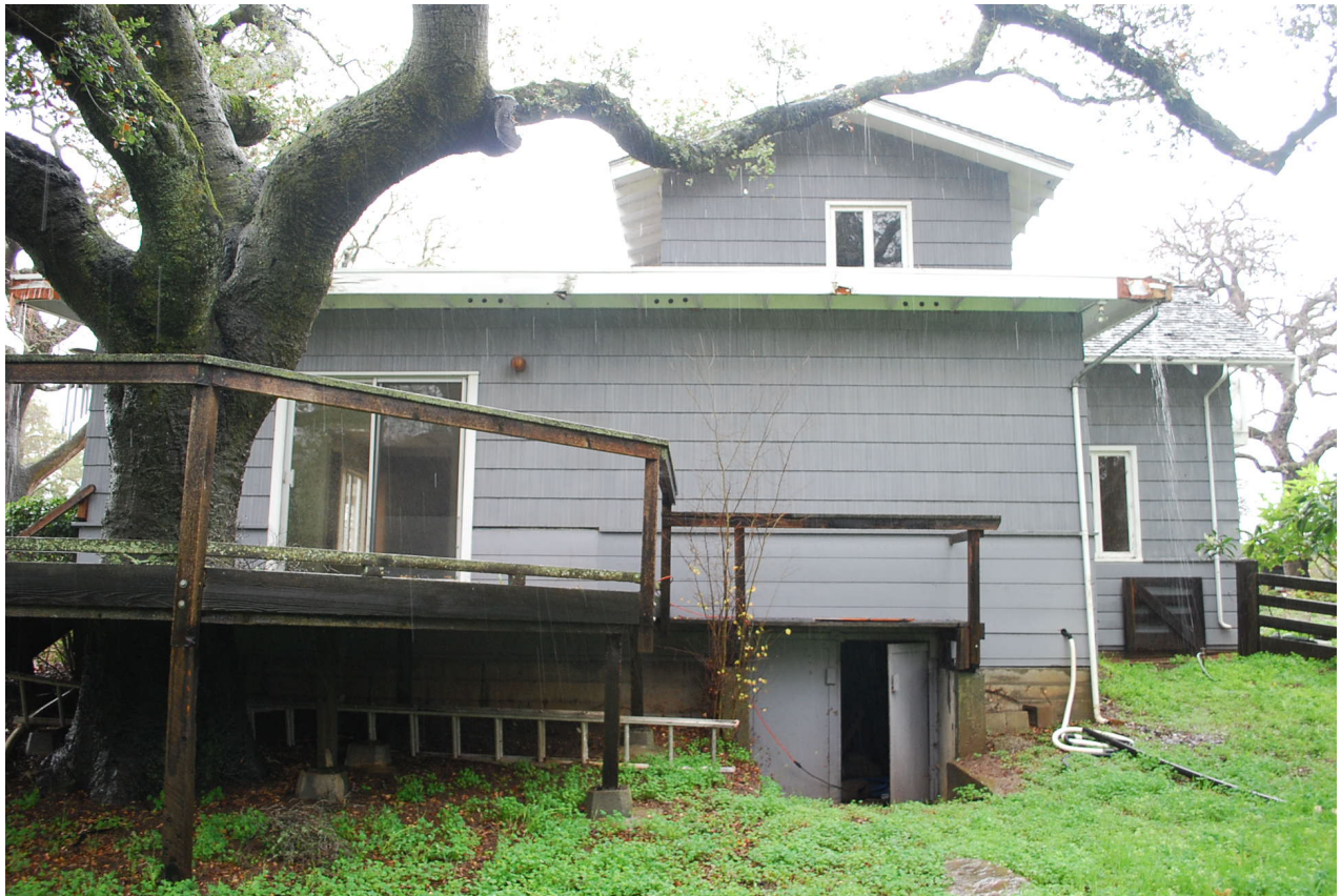
South facade. Most of what is seen here is an addition of unknown date. The old part of the house is at far right. To the left an aluminum sliding door opens onto a deck.
